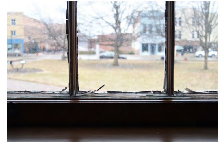
Deteriorating windows on the Vandalia statehouse. Fundraising is underway to restore all the courthouse windows.
